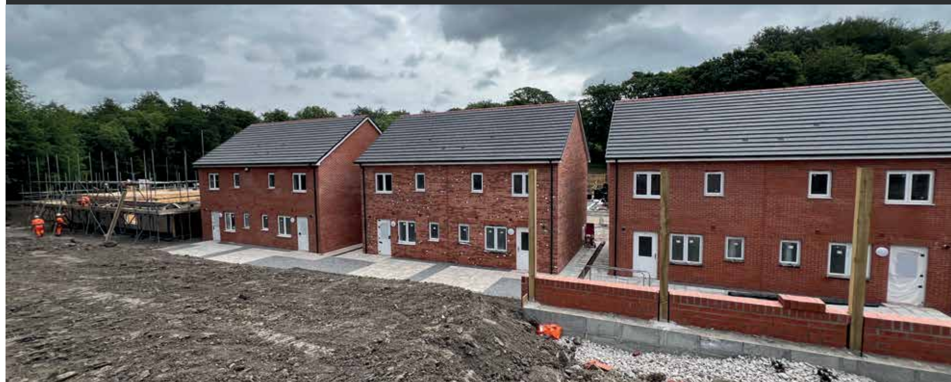
The Eaglesbush development is coming on well with stage one due to be complete by August
